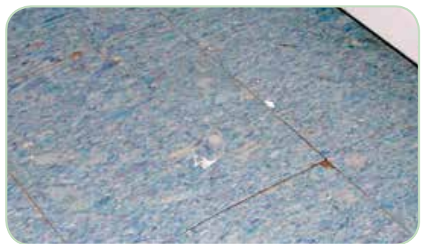
Typical old vinyl floor tiles that might have asbestos in the backing material
