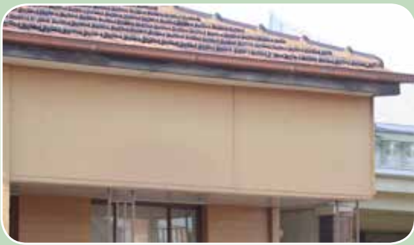
Asbestos cement sheeting in eaves
