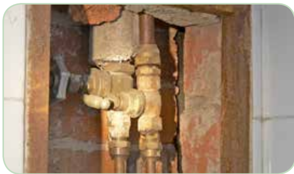
Friable asbestos lagging on pipes
